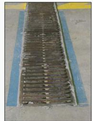
Coal & Ash Contaminated Water
